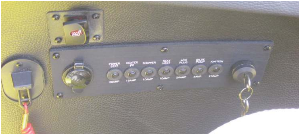
Figure 2-13. Circuit Breaker Panels
