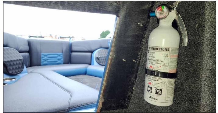
Example of a properly mounted portable fire extinguisher.
