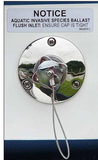
Ballast tank flush kit connector, located on starboard side of the transom.
