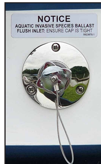
Ballast tank flush kit connection, located on starboard side of the transom.
